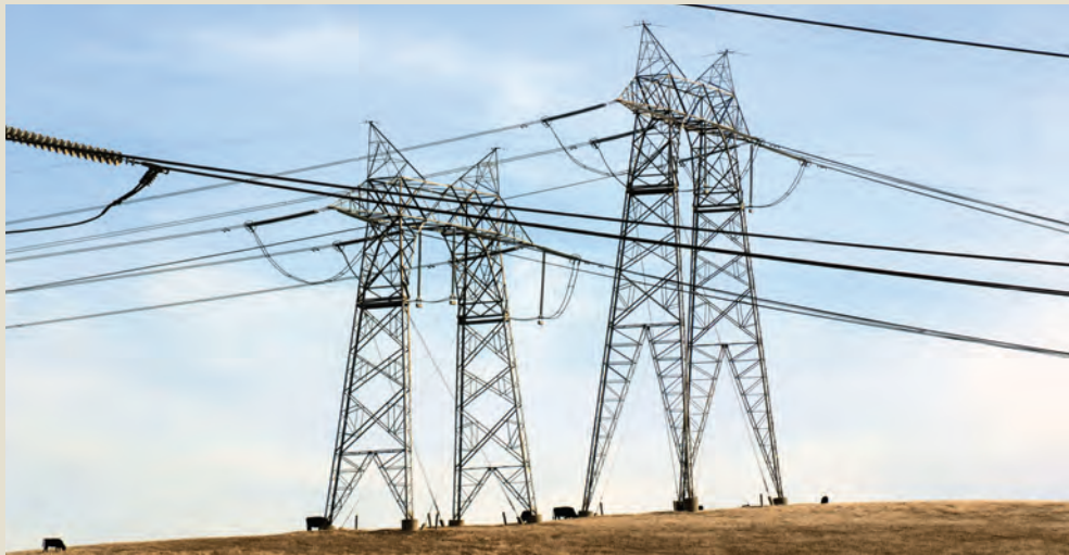
Source: Pacific Gas and Electric Company.
